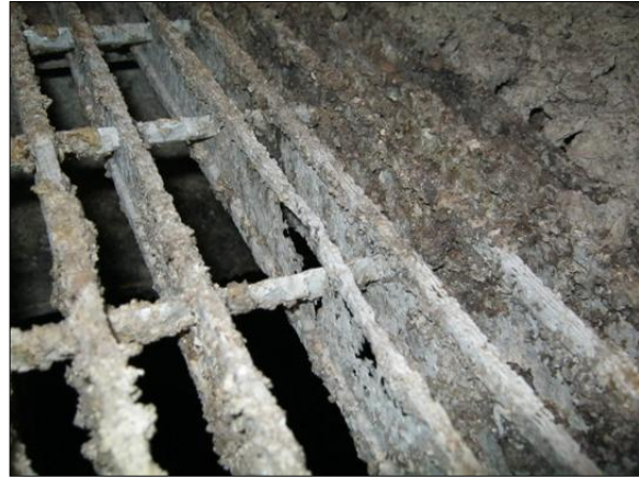
Photo 18. Small holes and perforations in thin members of grating.
