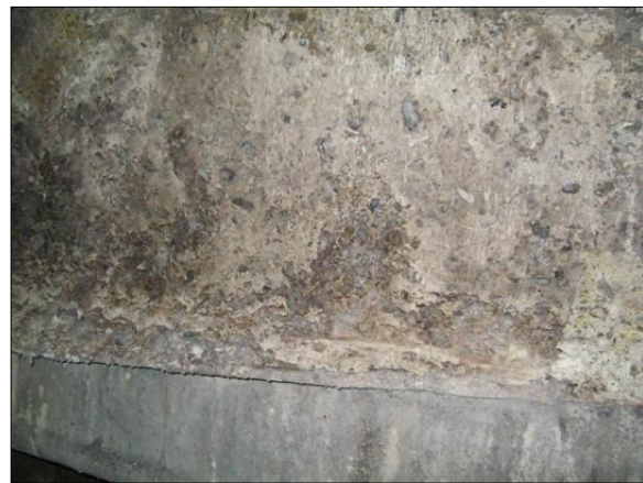
Photo 10. PVC T-Lock liner delaminating away from deteriorated concrete.
