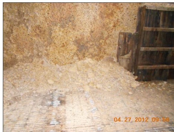
Photo 2. View of Influent Room looking at south wall showing pile of deteriorated concrete around perimeter of grating.
