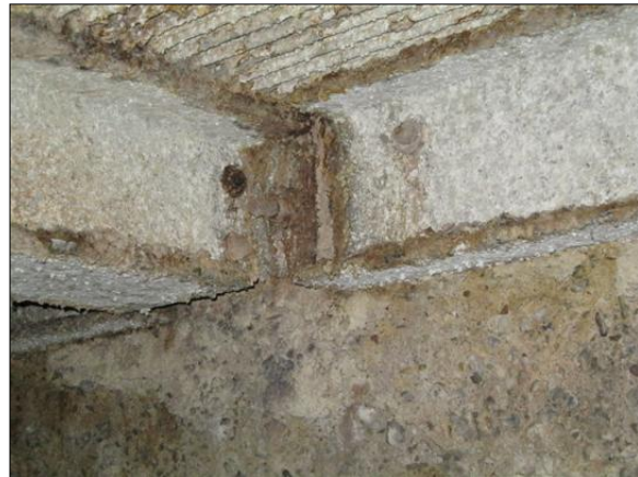
Photo 20. Aluminum beams and rafters covered with aluminum oxide but still sound.
