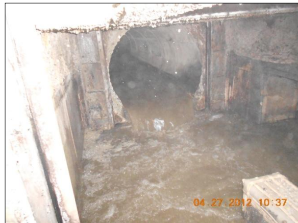
Photo 16. Concrete deterioration around west inlet penetration.
