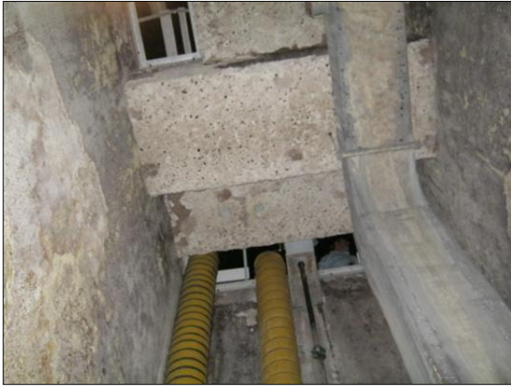
Photo 3. View of Influent Room looking at roof showing deteriorated concrete on walls and roof.
