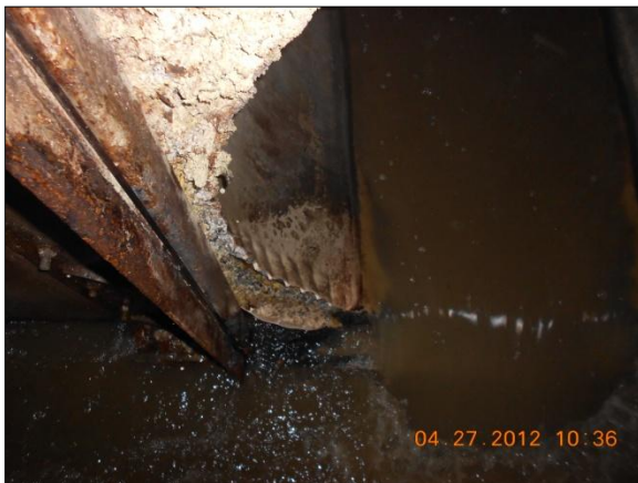
Photo 15. Concrete deterioration around south inlet penetration and T-Lock liner peeling on inlet pipe.
