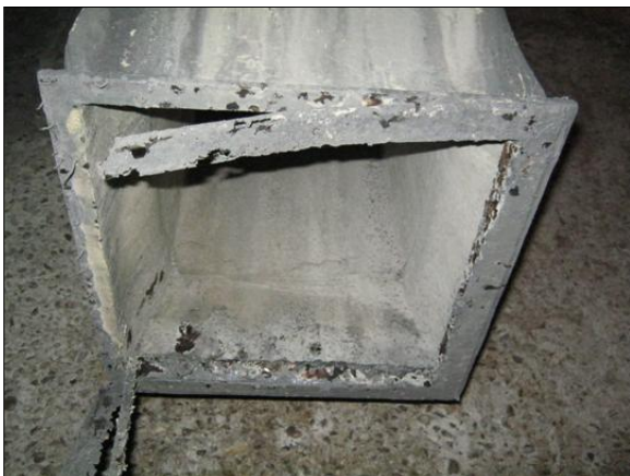
Photo 25. Screen to HVAC ducting missing.
