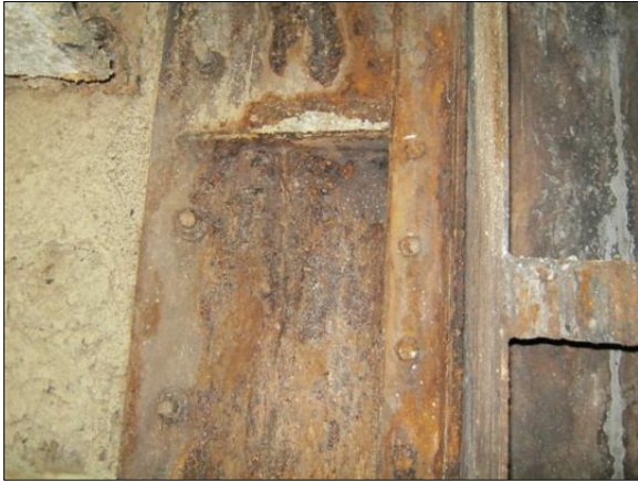
Photo 21. Surface corrosion and pitting on south sluice gate mounting/guide plate.
