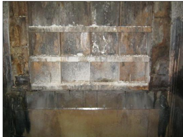
Photo 24. West sluice gate with corrosion similar to south sluice gate.
