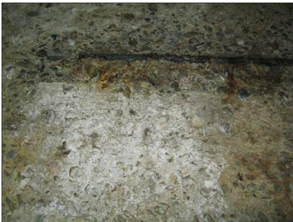
Photo 7. Exposed stray reinforcing steel on south wall.
