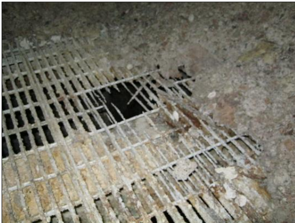
Photo 19. Patch of grating beneath HVAC ducting corroded through.
