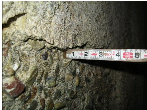
Photo 6. Side profile of concrete wall deterioration showing approximately 1.75 inches of concrete lost.
