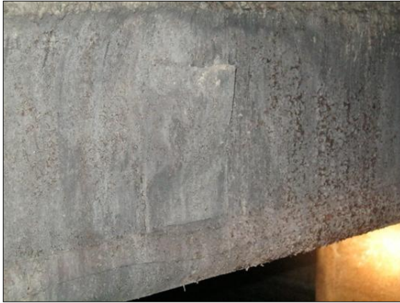
Photo 11. T-lock liner away from termination edge in good condition.
