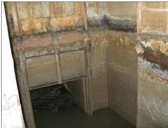
Photo 13. PVC T-Lock on walls of flow channel in good condition.
