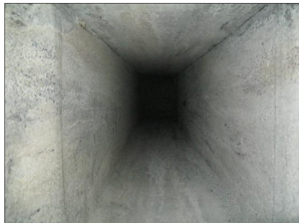
Photo 26. HVAC ducting appears to be open.
