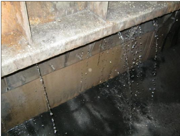
Photo 23. South sluice gate leaking approximately 2 to 5 gpm.
