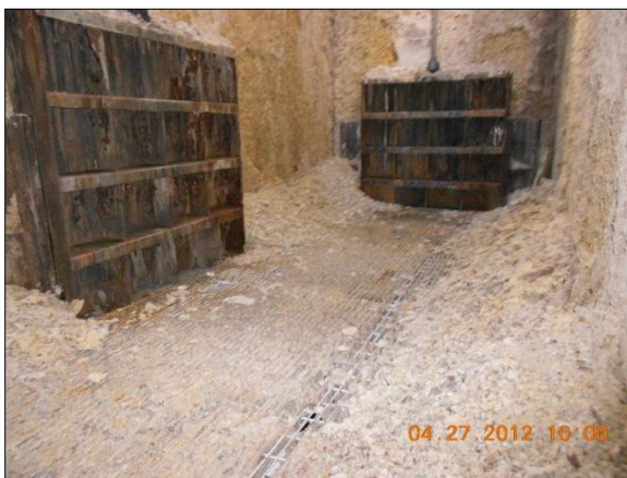
Photo 1. View of Influent Room looking at west wall showing pile of deteriorated concrete around perimeter of grating.
