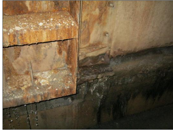
Photo 22. Surface corrosion and pitting on south sluice gate.
