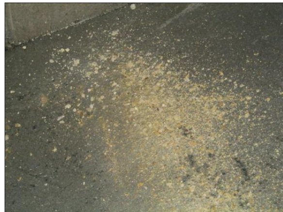
Photo 14. Minor erosion corrosion on floor of flow channel.
