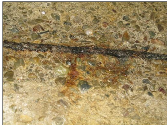
Photo 8. Detail of exposed stray reinforcing steel on south wall.
