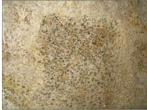
Photo 4. Pressure-washed area showing medium and large diameter aggregate, but no reinforcing steel.
