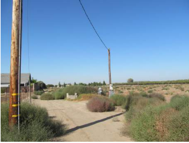
7. View of the well and pump equipment located at the southwestern portion of the property.
