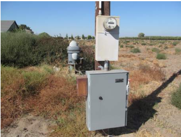
9. View of the well and pump equipment located at the southwestern portion of the property.
