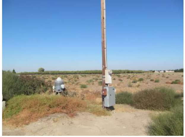
8. View of the well and pump equipment located at the southwestern portion of the property.
