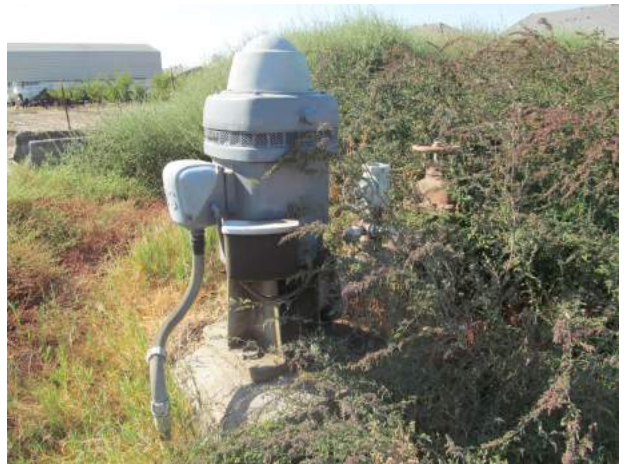
10. View of the well and pump equipment located at the southwestern portion of the property.
