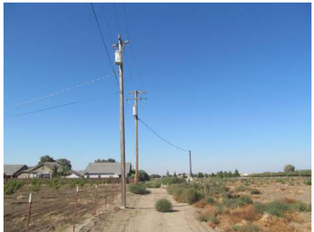
6. View of the pole-mounted transformers located at the southwestern portion of the property.
