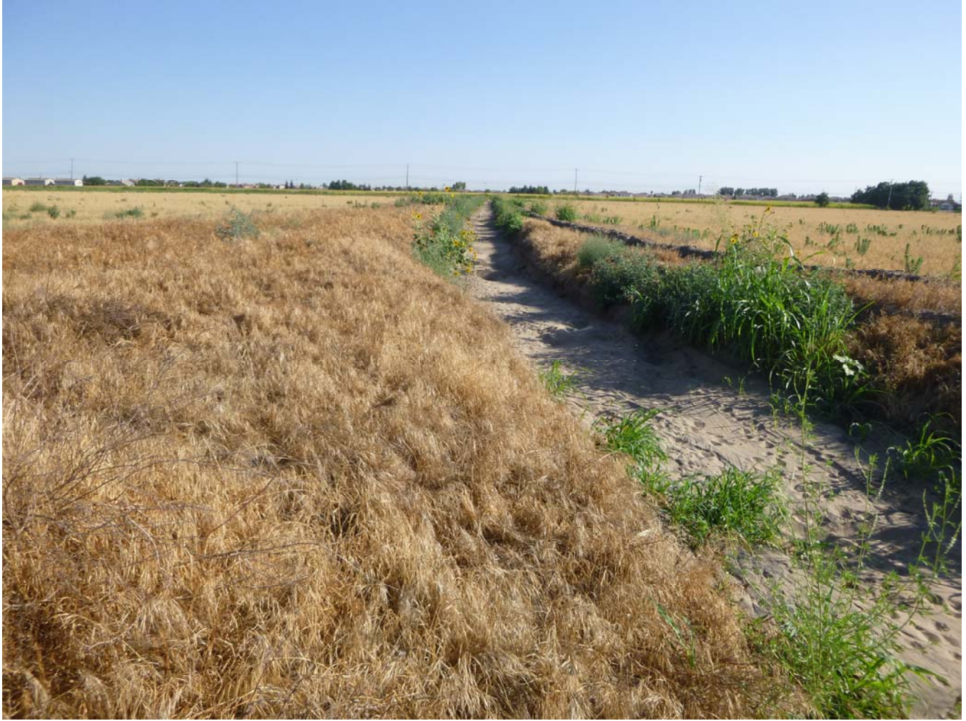
Photo 5. View of drainage ditch located in the middle of the Project Area, looking north (ditch runs north-south).
