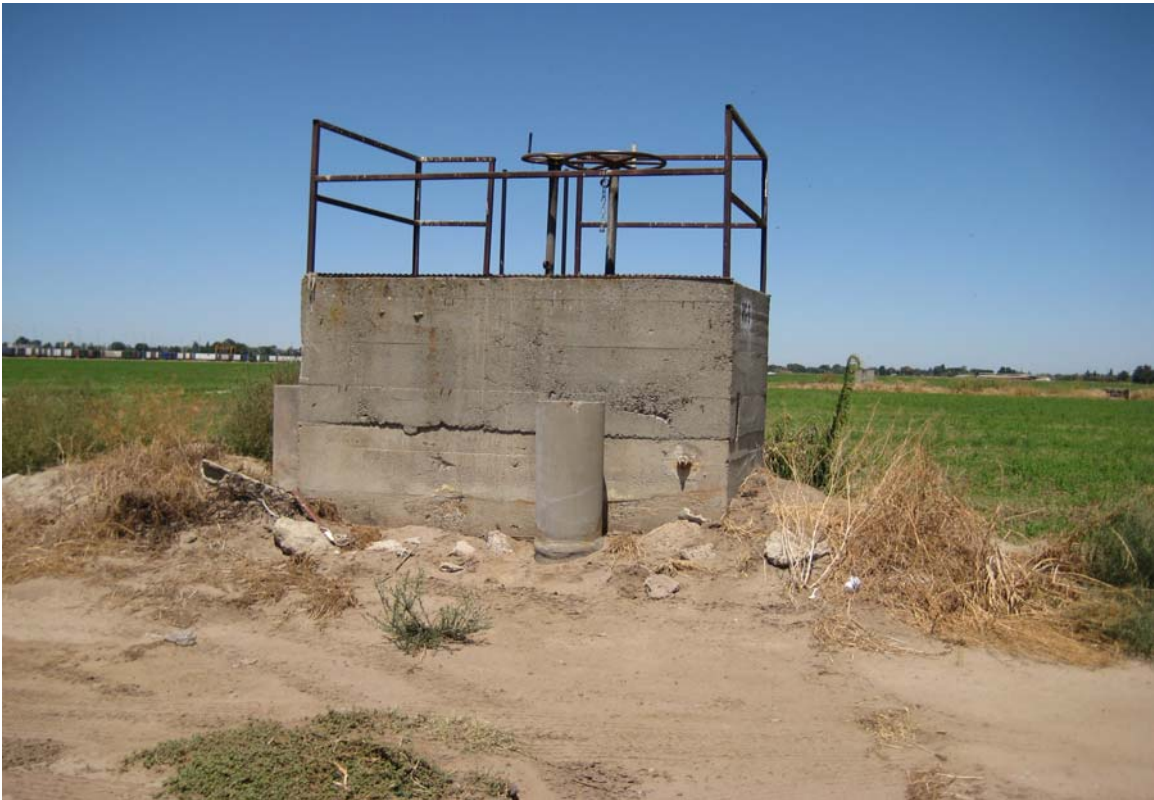
[12] IRRIGATION PUMP STATION: (Facing North) Flood irrigation distribution station.
