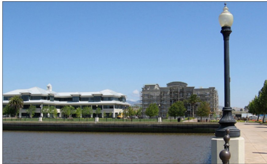
A 102-room motel (right) rises next to a new office building on the Suisun City waterfront.
