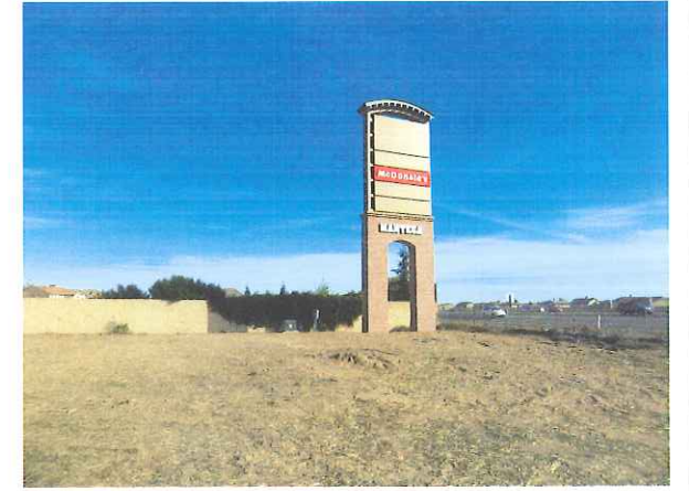
PHOTO 5: Sign and associated electrical panel and pad-mounted transformer in southeast corner of the site.
