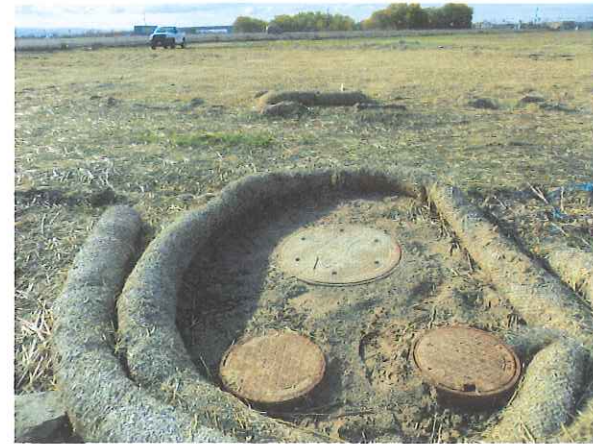
PHOTO 8: Storm drain filtration unit cover noted near southeast corner of the site.
