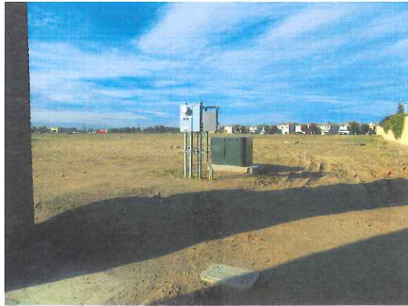
PHOTO 6: Close-up of electrical panel and pad-mounted transformer associated with large sign noted in photograph 5.
